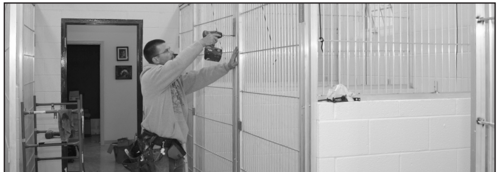
Co-owner Tony Hostutler installs cages at the new Broadview Acres Country Canine Resort.
